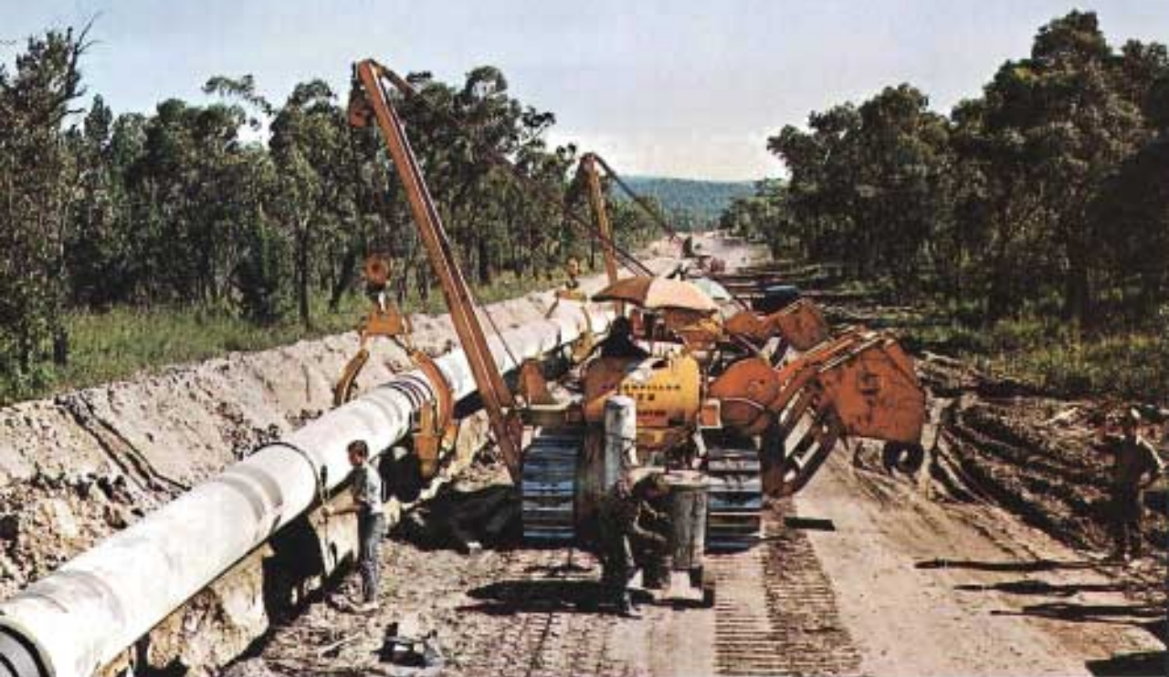
Crude oil pipeline under construction near Longford in Gippsland. Esso (Australia) Ltd
